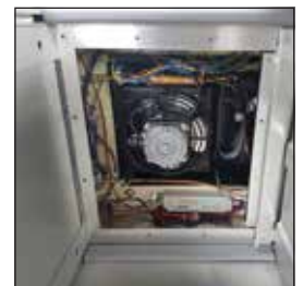
A5. Condenser compartment
