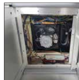
A5. Condenser compartment
